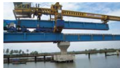
Launching of Griders at the Railway bridge connecting Idapalli and Vallarpadam, RVNL.
