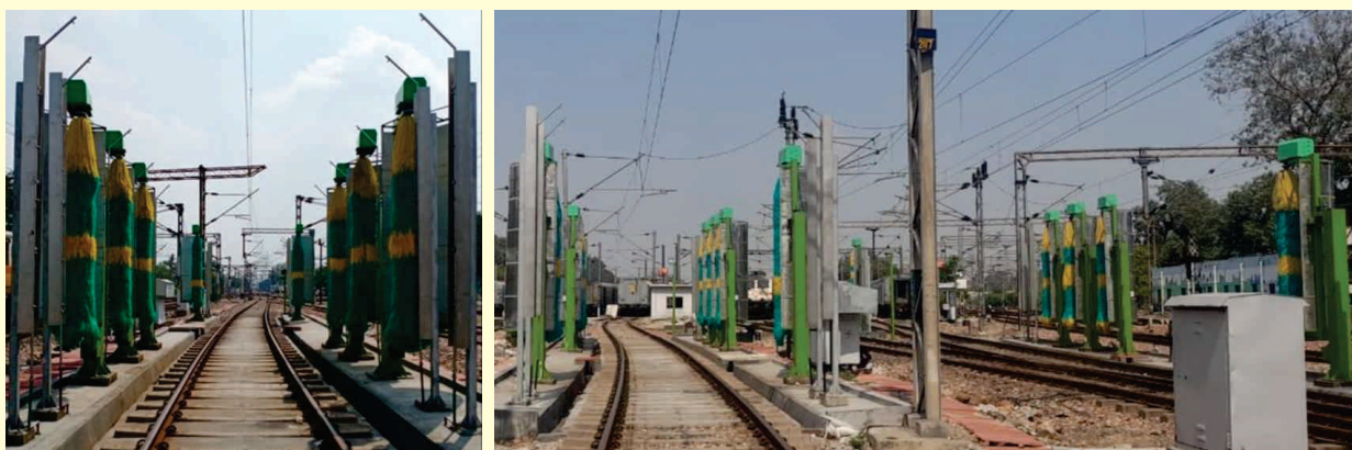
Automatic Coach Washing Plant at DLT complex, New Delhi
