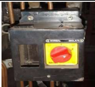
Fig. 18(9) Kernex: Kavach Isolation switch at Pn.panel
