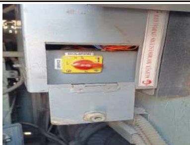
Fig. 18(12) Kernex: Kavach Isolation switch
