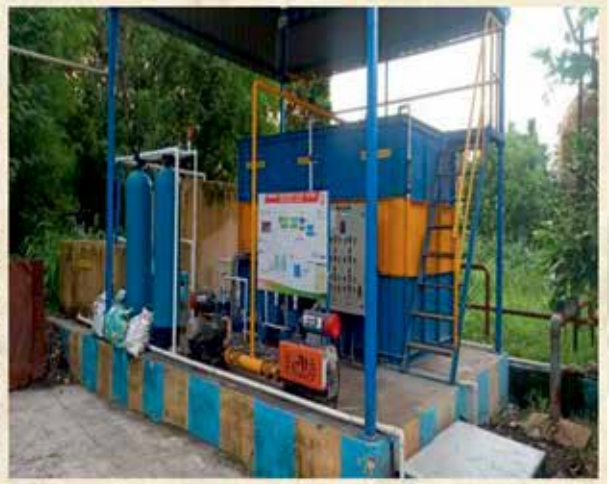
STP at Perambur Workshop
