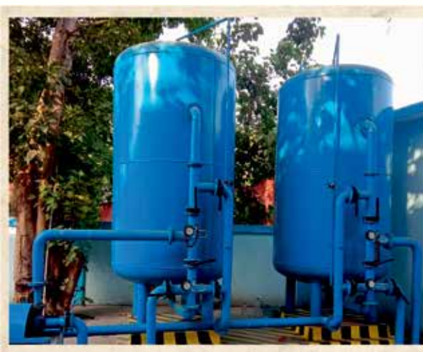
WRP installed at Patna
