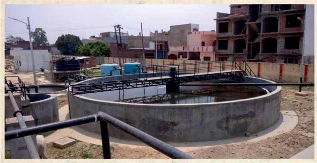
Sewage Treatment plant of capacity 1.6 MLD is operating in Research Design & Standards Organisation (RDSO)
