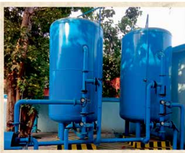
WRP installed at Patna
