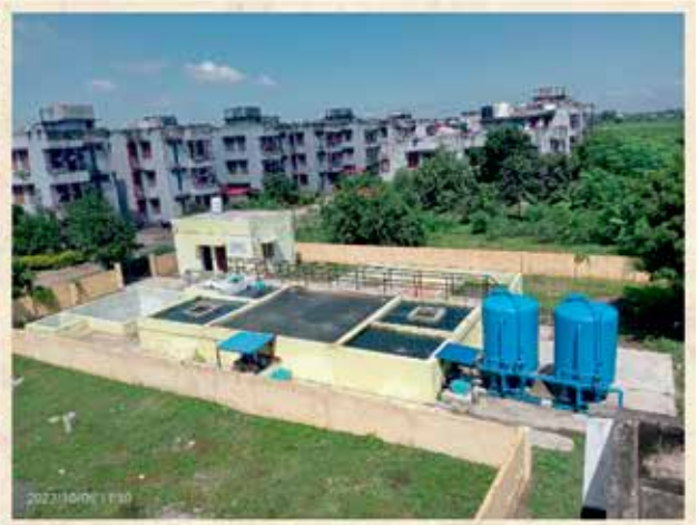
WRP installed at Harnauth Work shop
