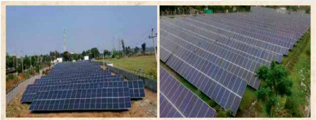
Solar Plant Feeding into Traction Sub-Station Installed at Diwana
