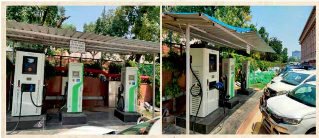
EV Charging station installed in Railway Board, New Delhi
