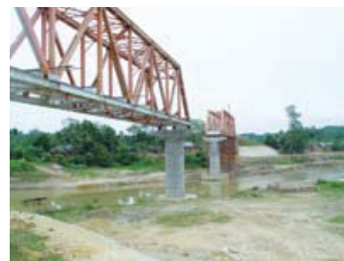
Railway bridge under construction – Kumarghat - Agartala new line (National Project), Northeast Frontier Railway.
