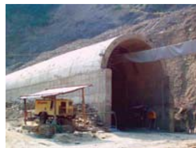
Tunnel construction work – Kumarghat – Agartala new line (National Project), Northeast Frontier Railway.
